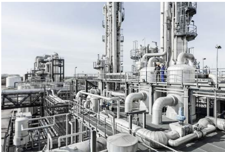
Figure 11: Example of a process plant
